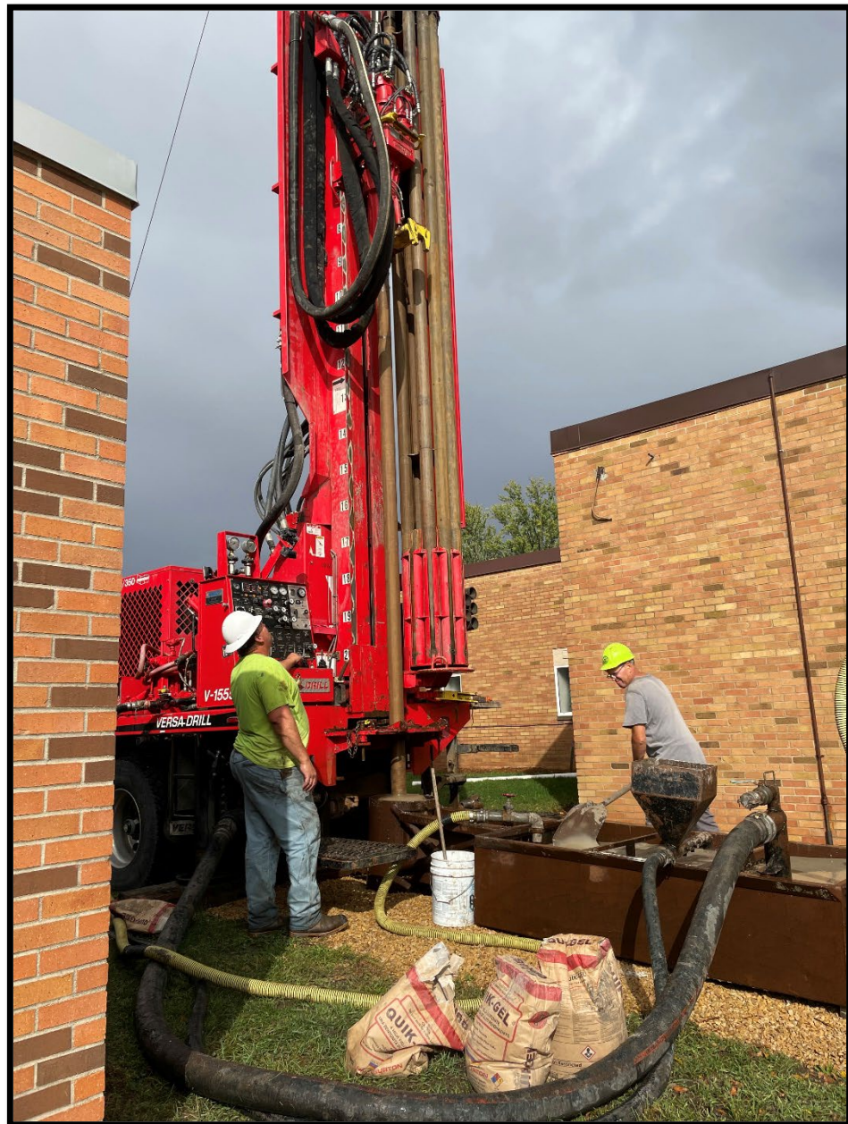
Figure 9. Well Contractors Drilling into Municipal Well to remove debris before sealing. Photo Credit: Holly Bushman
