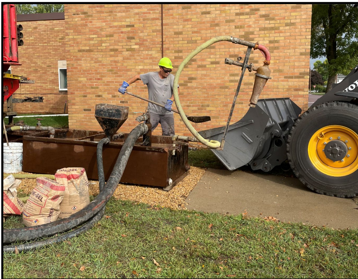
Figure 8. Well Contractor removing sand and sediment build up from drilling the well. Photo Credit: Holly Bushman
