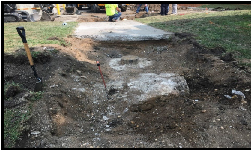
Figure 7. Old Municipal Well #1 Before Well Sealing. Photo Credit: City of Le Center
